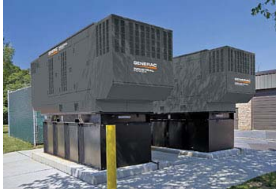
Paralleled Generator Application
